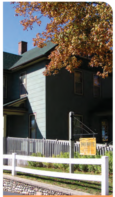
Through a grant from an affiliate fund, the Iowa Falls Historical Society was able to re-roof the Dow House.
